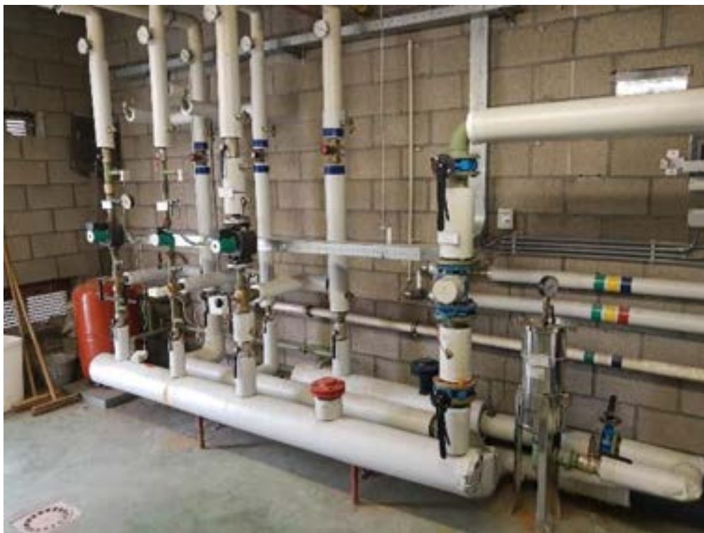
Figuur 25: Stookinstallatie Boortmeerbeek
